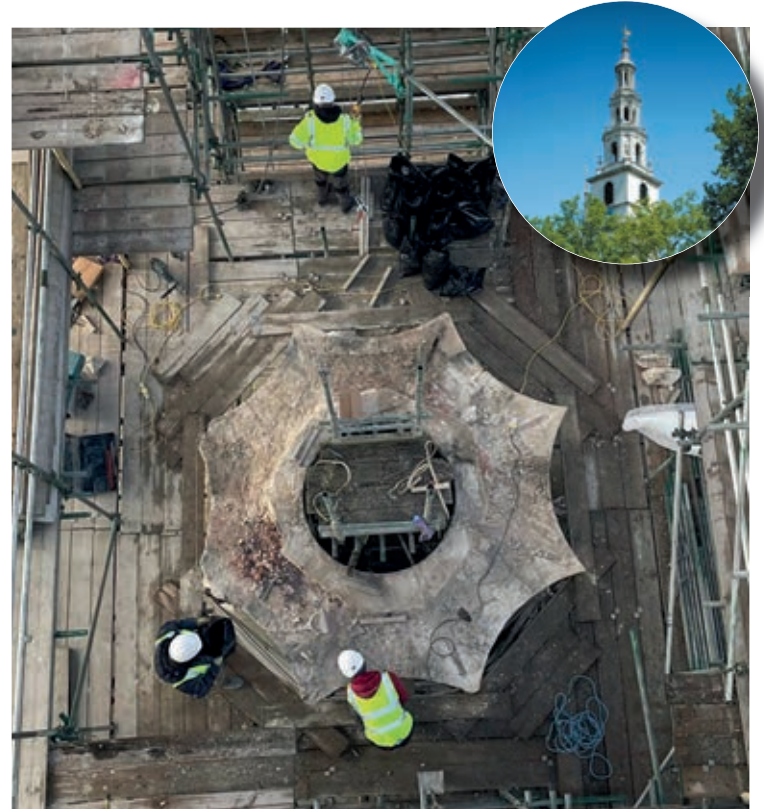
RESTORATION: Specialist teams at work dismantling damaged steeple ahead of rebuilding work due to start in May this year. Inset, the steeple before work began
